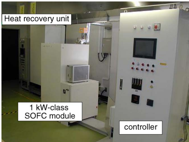
Fig. 3. Features of 1 kW-class demonstration co-generation system.
